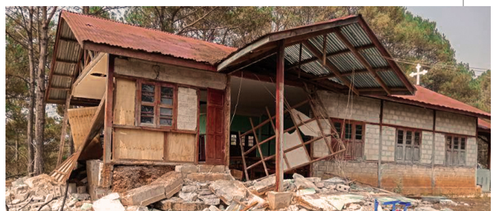
A church in Myanmar damaged by last month's devastating earthquake
